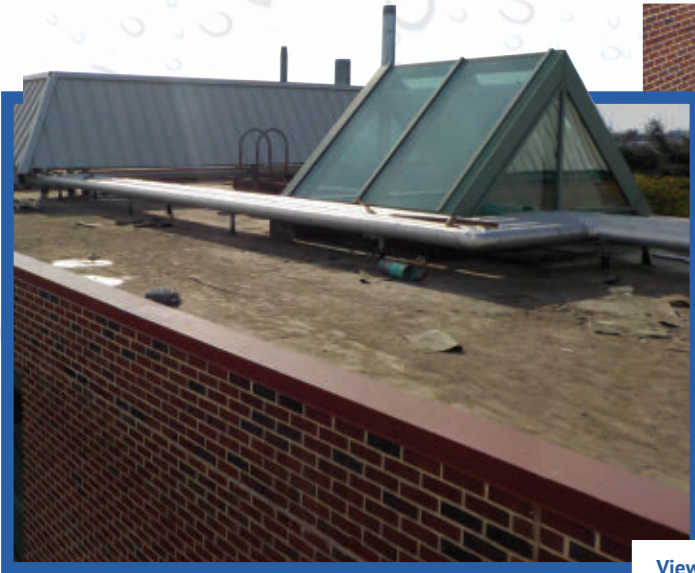
View of the PWD roof during the removal of the original EPDM system
