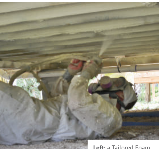
Left: a Tailored Foam crewmember applying SPF to the subfloor; Right: the spray foam created a moisture barrier for the home, which was nearby the water
