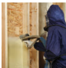
ON THE COVER p36 Best practices for the installation of SPF, like the PPE seen in our cover photo, are industry-wide priorities. PHOTO COURTESY of Icyne
