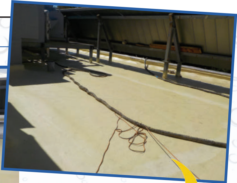
During the foam application portion of the project, the JJD Urethane crew installed two inches of SPF
